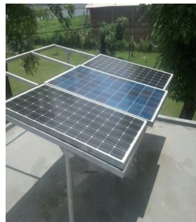
Figure 2. Solar photovoltaic panels at PLTMG-CNG Bawean.
