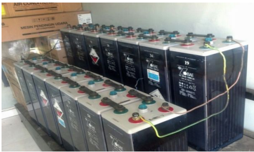
Figure 3. Batteries used for power storage from photovoltaic panels
