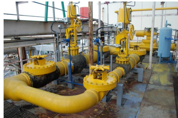
Figure 3. Plant piping and instrumentations after retrofit
