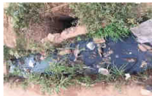
Figure 2: Waste water flowing on the pavement
