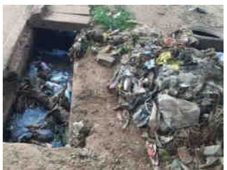
Figure 3: Rainwater and sewage mix
