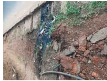
Figure 5: Waste water flowing on the pavement
