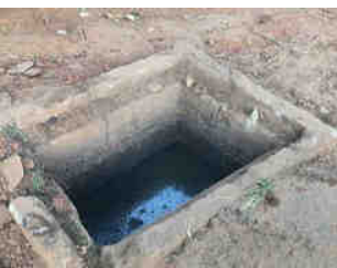
Figure 4: Open and obstructed concrete manholes
