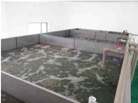
Fig. 15 Clear water test run
